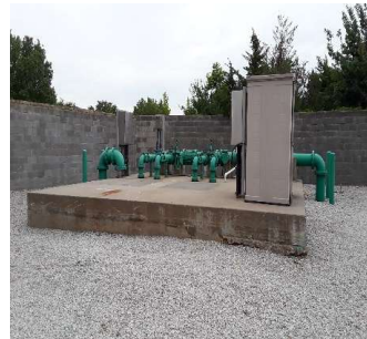
13 Lift Stations Maintained
